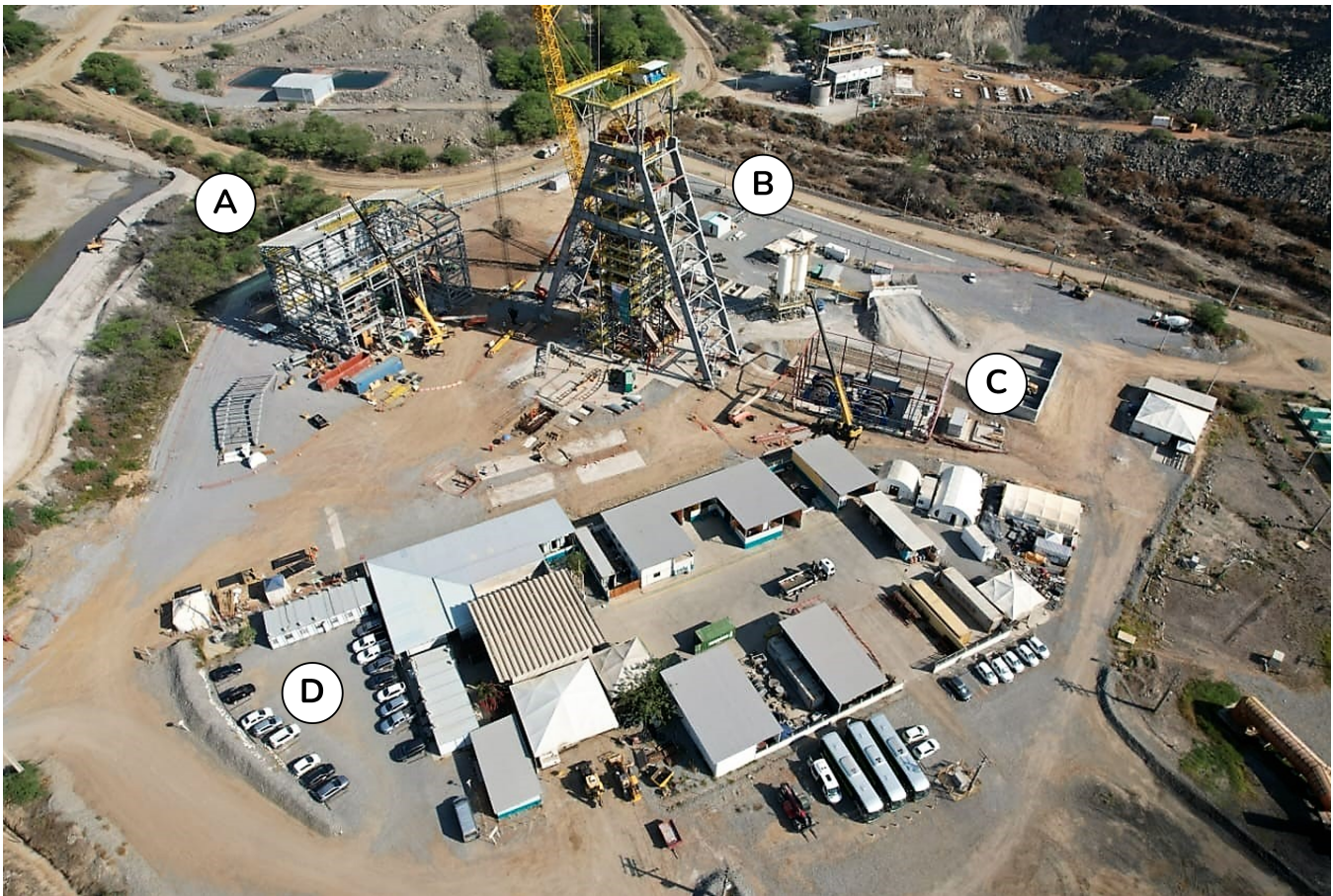
Figure 1: October 2023 aerial view of the Caraíba Operations shaft project, including (A) the permanent rock and personnel winders, (B) the completed shaft headframe, (C) the stage winder foundation, and (D) engineering and administrative buildings.
