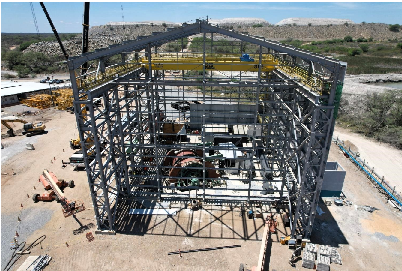
Figure 2: Progress on erection of the permanent rock and personnel winder building (October 2023).
