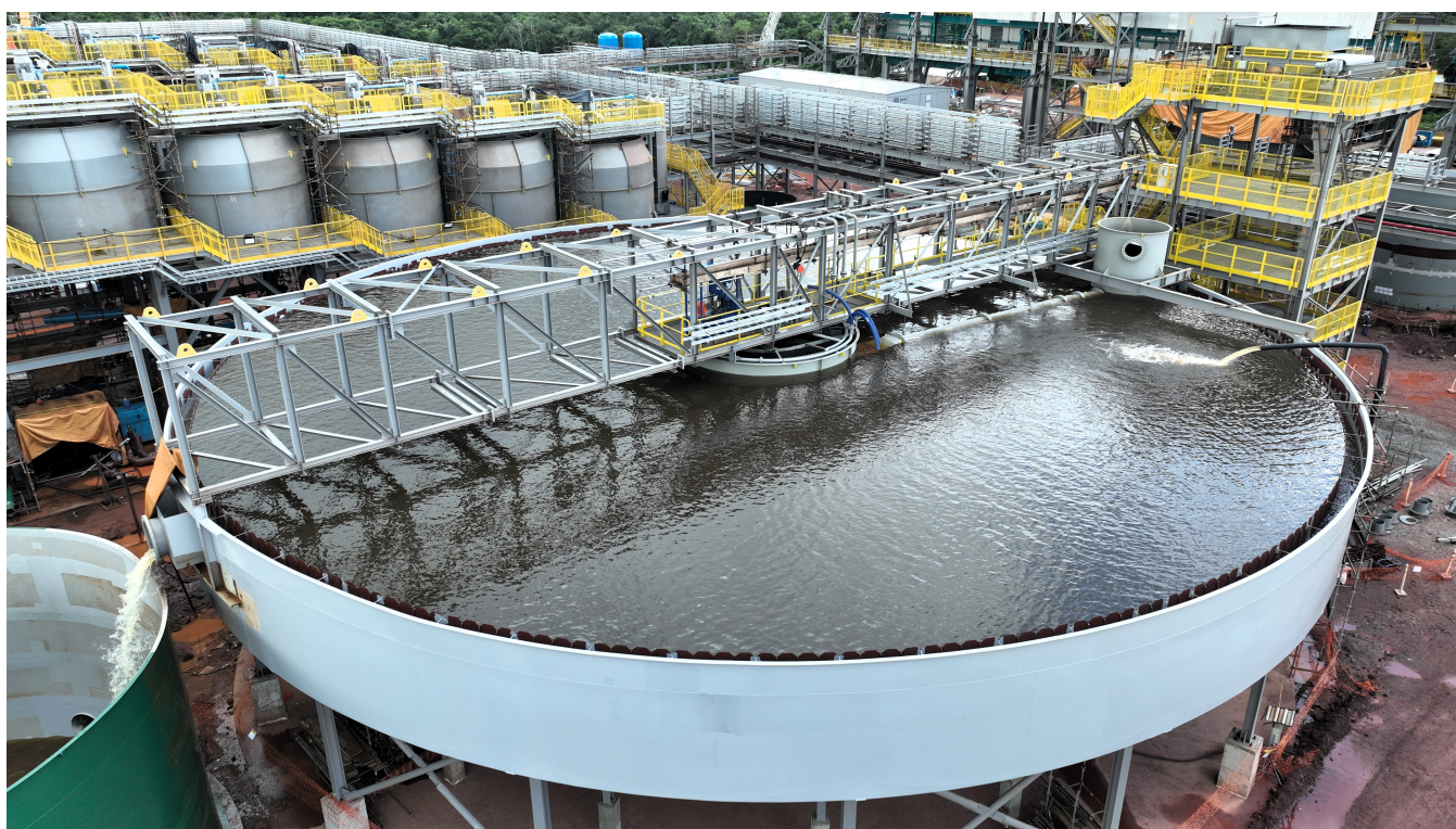
Figure 2: Tailings thickener at the Tucumã Project (May 2024).
