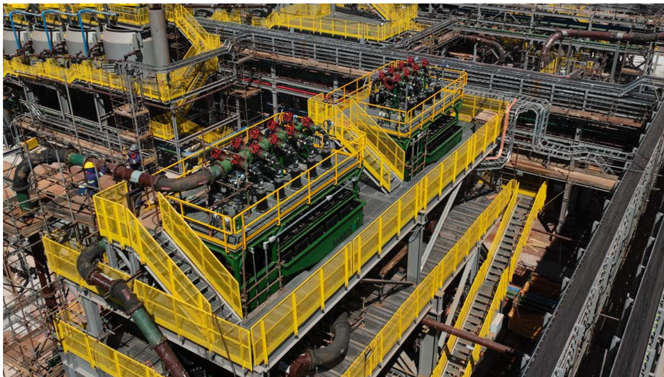
Figure 4: Completion and commissioning of Jameson flotation cells as of June 2024.
