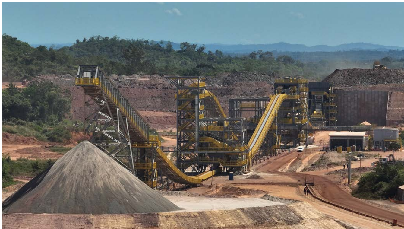
Figure 2: Completed crushing circuit with ~10,000 tonnes of crushed ore placed on stockpile (June 2024).
